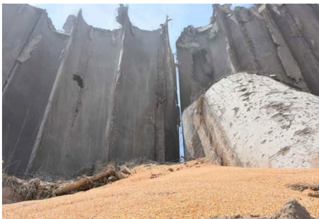
Destroyed grain silos in the port of Beirut, which handles the majority of Lebanese imports
